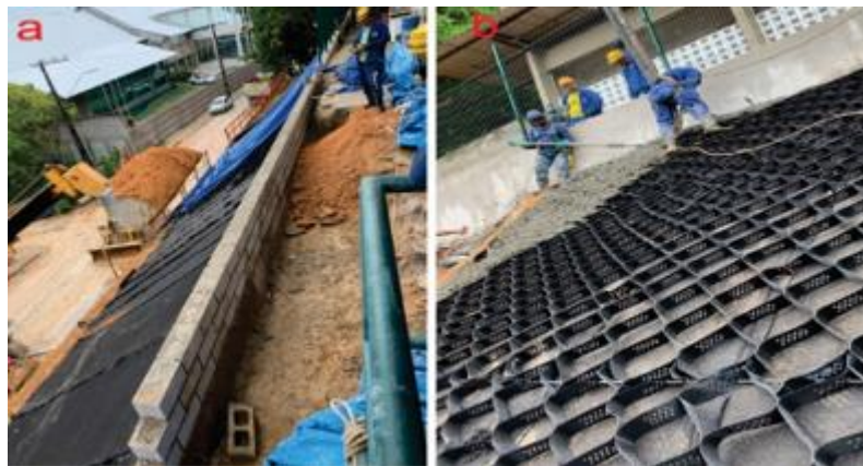
Figure 10 - (a) application of geotextile over the slope after compaction; (b) fixation of geocells and then application of machined concrete.
