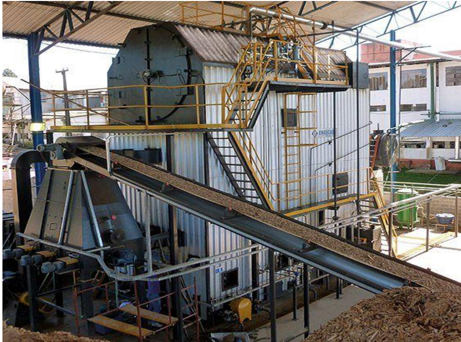
Figure 2. Steam Boiler of Biomass (ENGE CASS, 2017).
