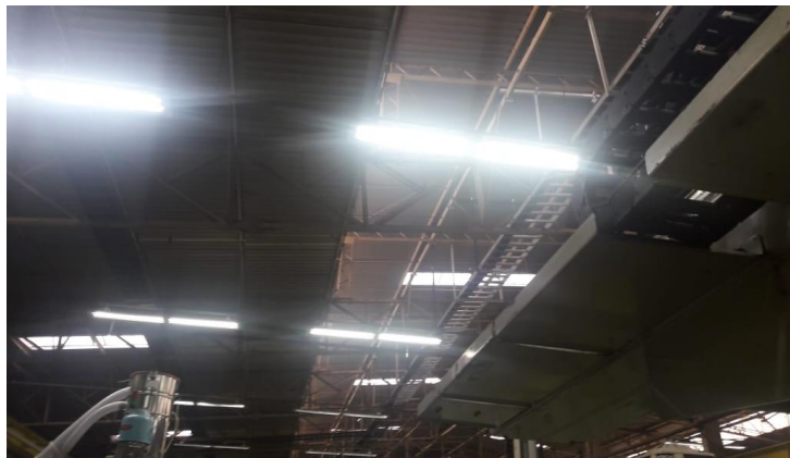
Figure 4. Shed Lighting Fixture.
