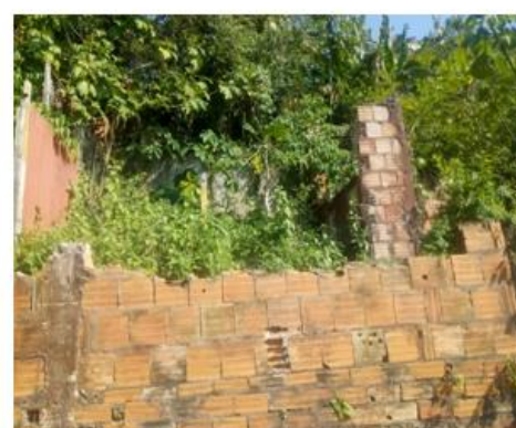
Figure 5: House destroyed by ground mass movement.
