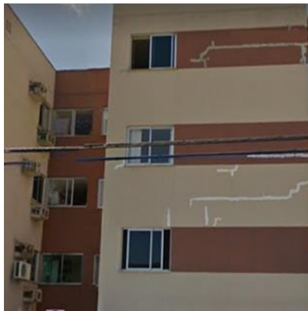
Figure 4 - Cracks in the facade of the residential building.
