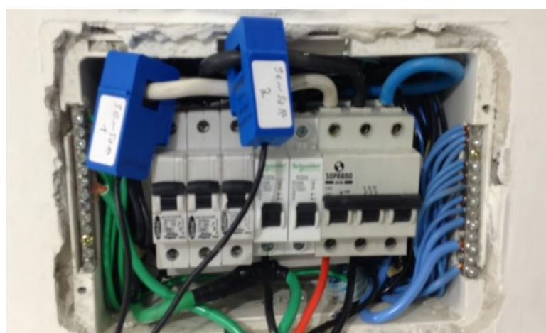
Figure 3. Integration of current sensors to the residential distribution board. SOURCE: Own author, 2019
