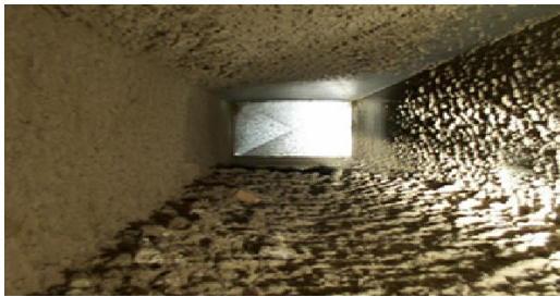
Figure 1. Ducts with dirt accumulation.
