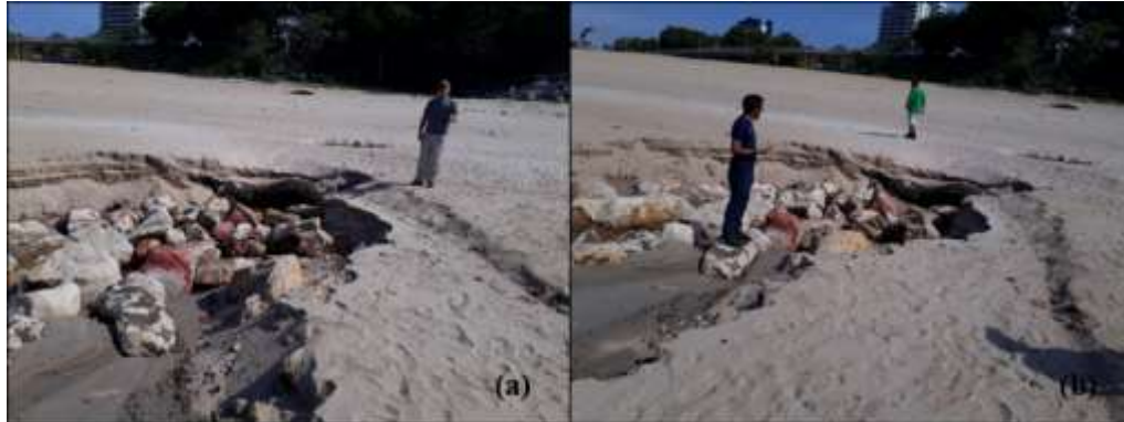
Figure 4: Features found on the transition surface of the embankment and natural beach, during the drought periods, in 2018 - a and b) Erosions with the appearance of the substrate rocks, approximately 2 meters wide, and 40 cm deep.
