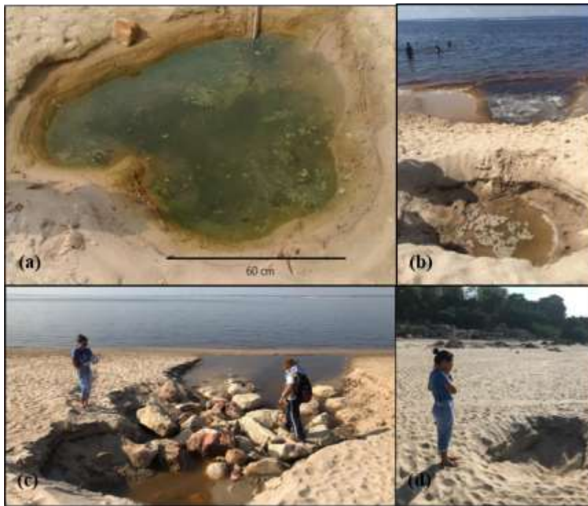
Figure 3: a) Abrupt depression / internal erosion feature in 2017 at the landfill; b) Erosion with the formation of pots on the artificial beach in 2018. c) Erosion on the natural beach, close to the beach line, of almost 6m in length in 2018. d) Cavities about 1 m in diameter in the embankment in 2018.
