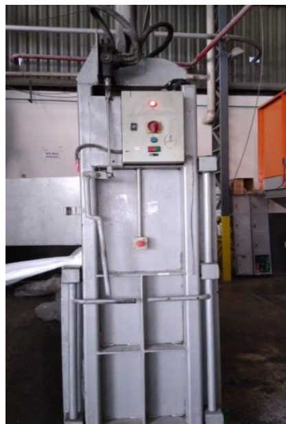
Figure 16 – Electrical Source: Author (2010)
