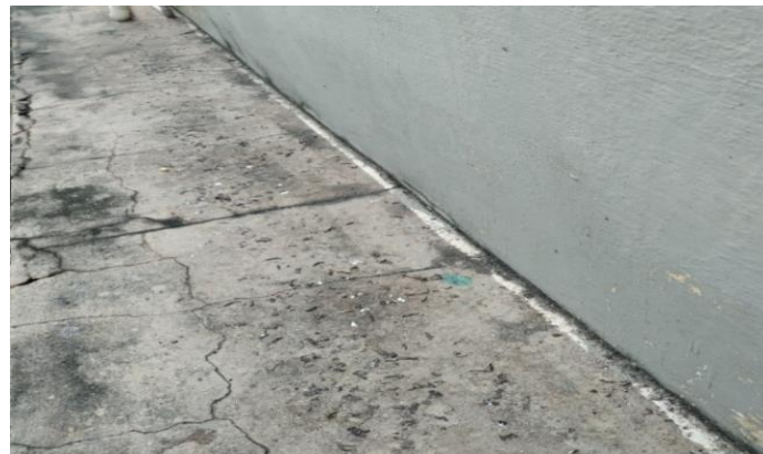
Figure 3 - Cracks in the sidewalk around the residence
