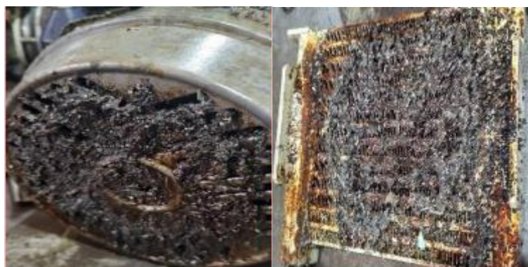
Figure 1. Pump cover and heat exchanger with excess dirt.
