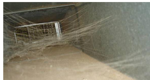
Figure 2. Insect presence housed in ducts.
