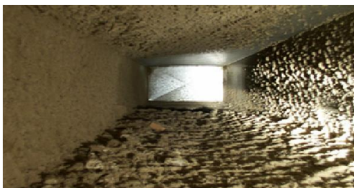
Figure 1. Ducts with dirt accumulation.
